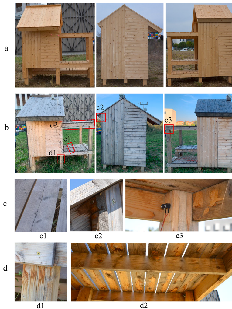
Fig. 7. Visual comparison of the wooden playhouse at construction (a) and after 21 months of exposure (b), showing early signs of weathering. Close-ups (c1–c3, d1–d2) highlight cracks, moisture-related staining, discoloration, and surface roughness in vulnerable areas.
